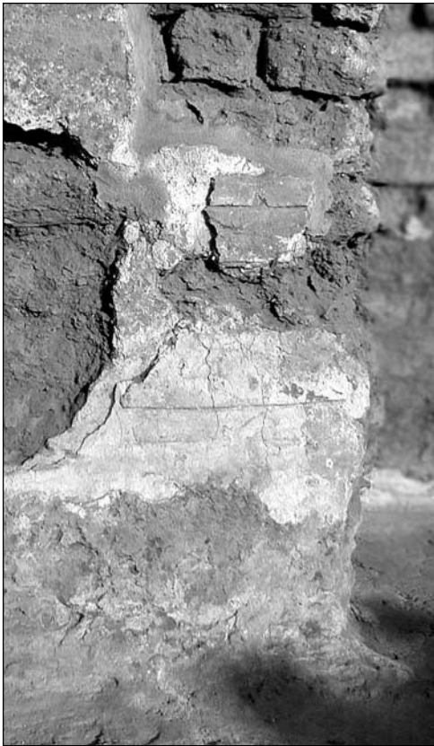
Fig. 4. Fragmentarily preserved stucco decoration on the second coating of plaster in the western arm (Photo D. Zielińska)
