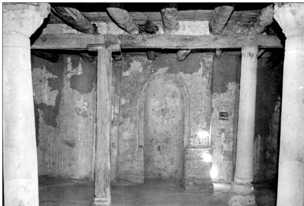
Fig. 13. Mosque: central room with mihrab on the first floor (Photo W. Jerke)
